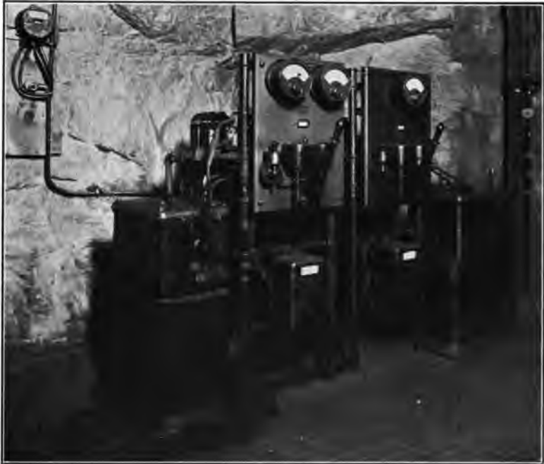
STEPHENSON MINE. PANELS FOR UNDERGROUND PUMPS
